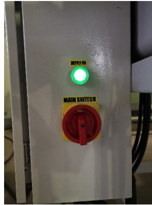
Fig.8 Main switch in the ON (1) position, with the SUPPLY ON button lit up, meaning the machine is turned on and ready for work.
